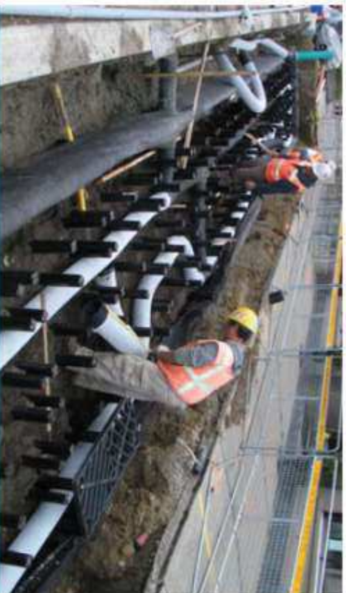
Figure 2.4.3: Installing the soil support system under the sidewalk on part of the Queensway in Toronto. (Source: Deep Root Inc.)
